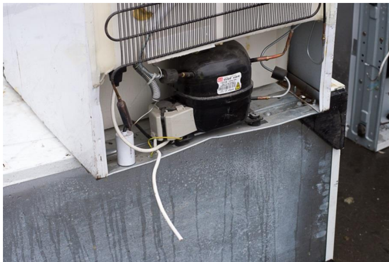
An example of a non- functional refrigerator: power -plug missing.
